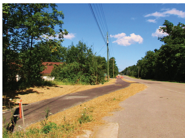
Construction began early last spring on Phase One of the non-motorized, recreational trail that winds through Young State Park and will eventually link Boyne City to Charlevoix and the growing Little Traverse Wheelway network throughout northern Michigan.
